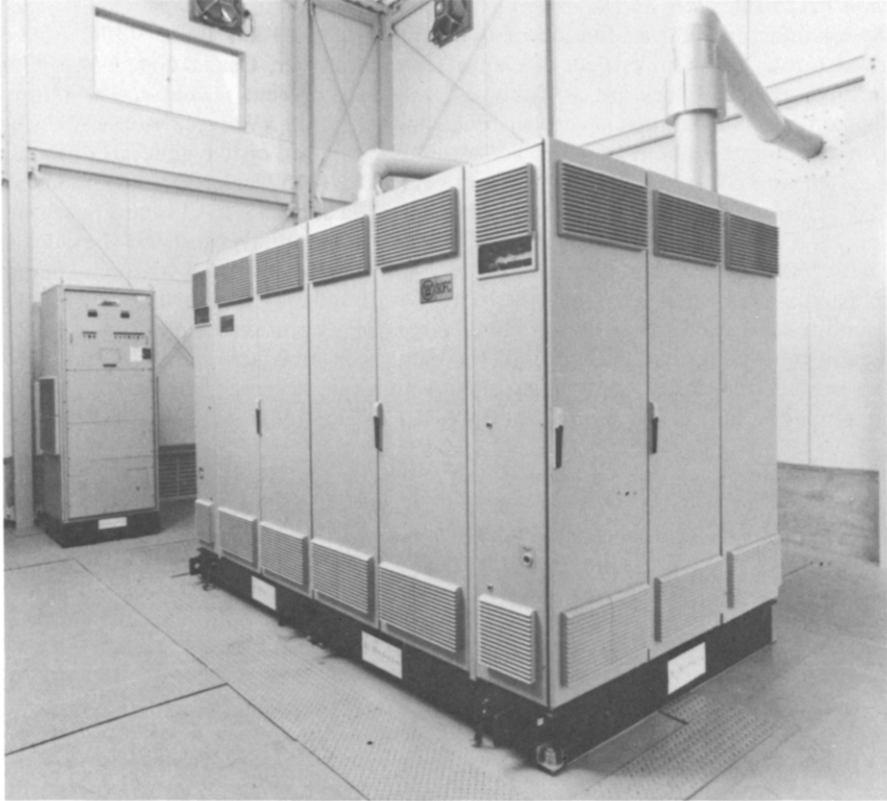
Fig. 2. 25 kW class SOFC system (first system).
